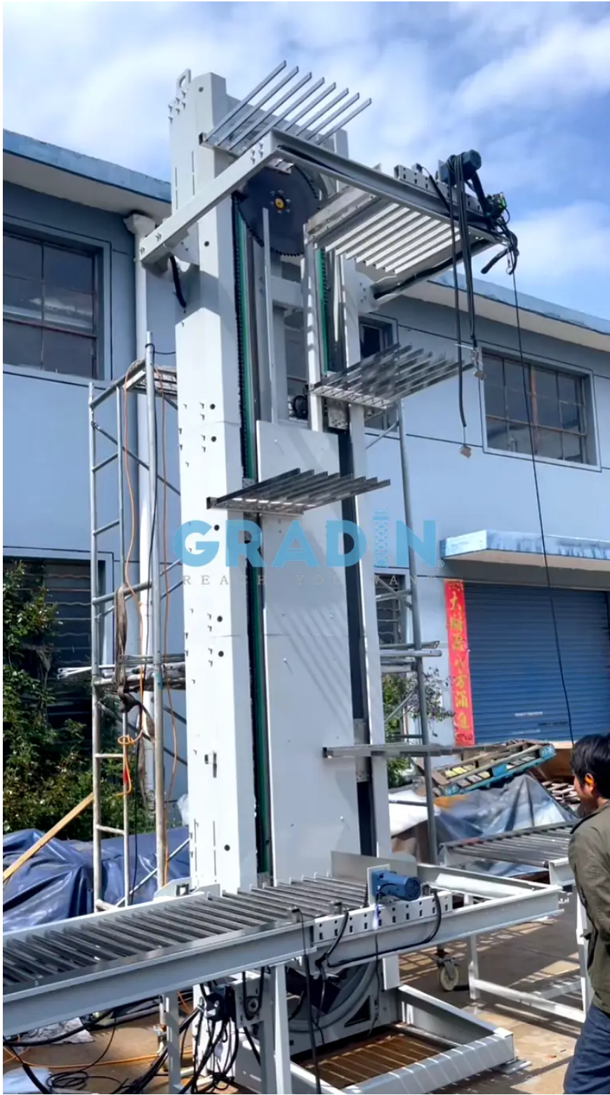
Figure 3: Integrated commissioning — technicians inspecting drive components from scaffolding, roller conveyor at inlet
