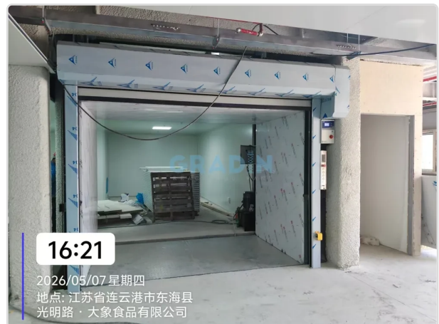
Figure 2: Stainless Steel Cabin and Roll-up Door
