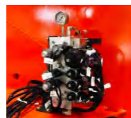
电气设备 electrical equipment
