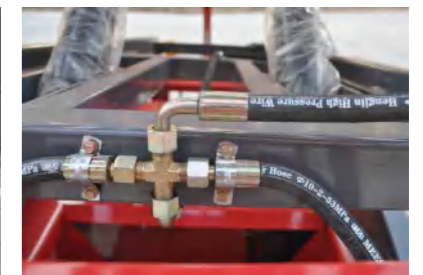
油管 C 型接头无渗漏 The C-type joint of the oil pipe has no leakage
