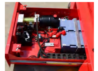
蓄电箱 Battery box
